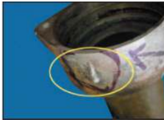
Figure 7: Non-operational damage - melted by torch
