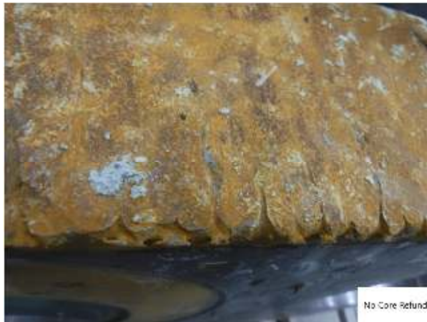
Figure 2 – The surface of the link has been welded and would be an example of an unsuccessful attempt to salvage, resulting in no core refund.
